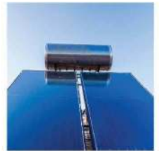
Solar Heater Point / Hot Cold Water Piping
